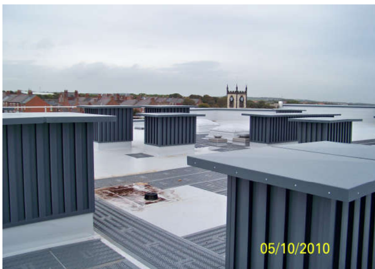
HPBT units supplied to Durham County Council. St John's Square, Seaham.
